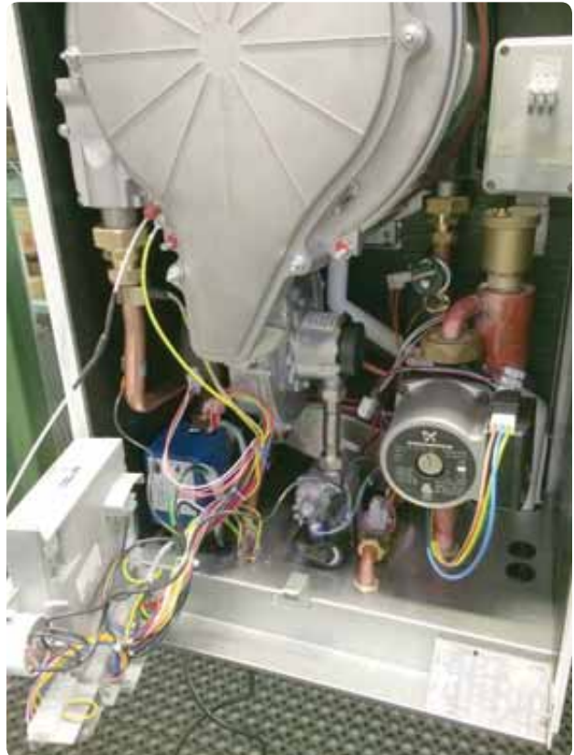
Figure 140 Boiler front panel removed
