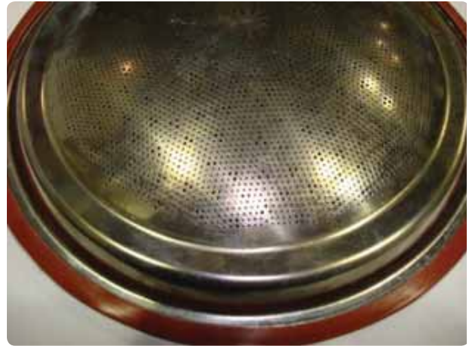
Figure 144 Inspecting exterior and cleaning the burner
