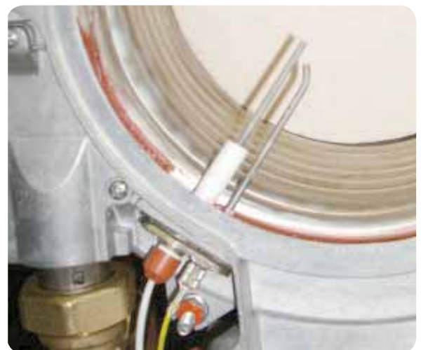
Figure 137 Inspecting ignition electrode
